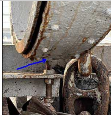
Excessive gap between brake band support screw
